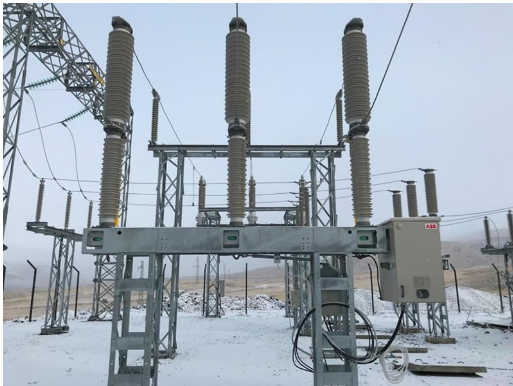
Figure 5-3: Site Substation for Power Grid Connection
